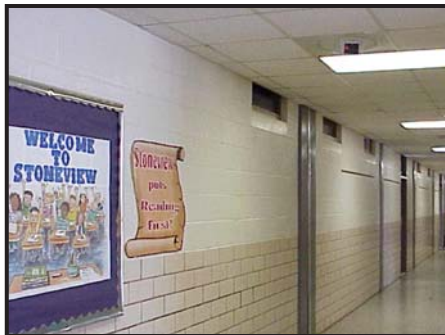
At Stoneview Elementary in Dekalb County, GA the RC200 ceiling mount is used for surveillance. The housing replaces a 2 x 2 ceiling tile, and can be manually rotated 360°.
